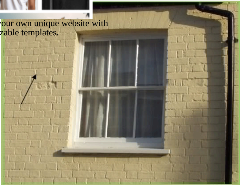
Damage to brickwork, caused by Knocker-Ups
